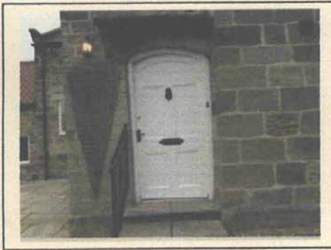
Photo 5 – Distortion to Entrance Door
