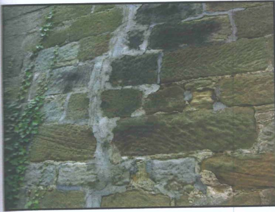
Detailed view of right hand gable crack
