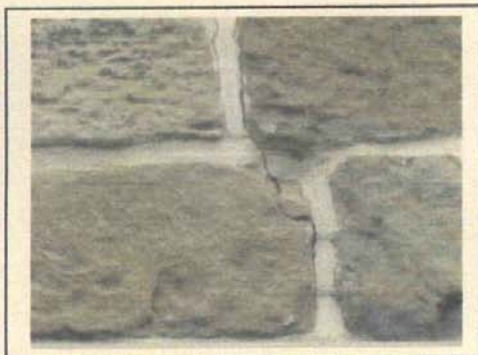
Photo 3 – Typical Damage to External Stonework
