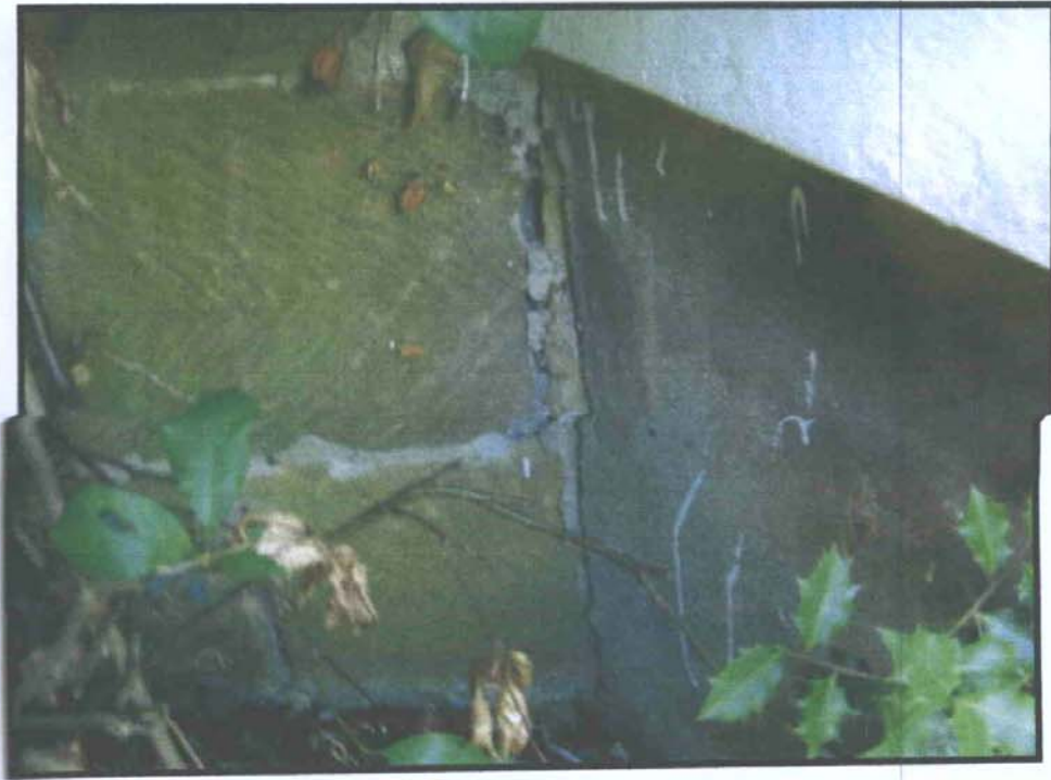
Cracked render to bay window lower wall
