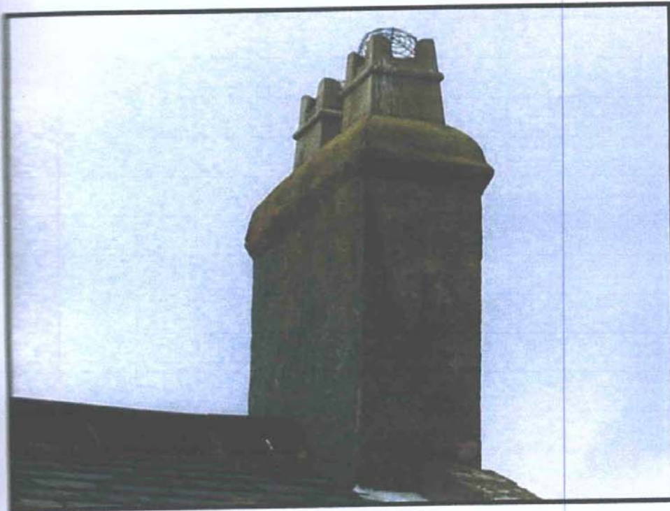
Right hand side chimney-stack leaning, and cracked and poor render
