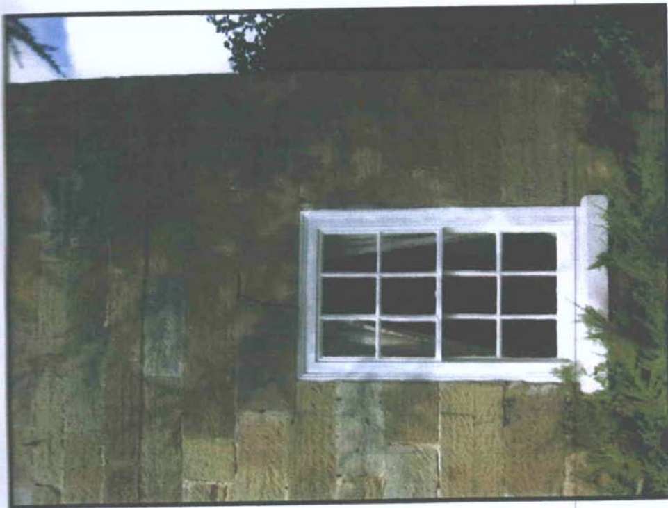
Left hand side gable with cracked lintel and cracking to wall
